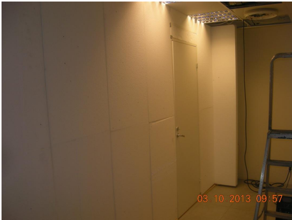
Figure 20. Photograph illustrating the right temporary Styrofoam wall in figure 19, which was shared by the two considered spaces and had a built-in door.
